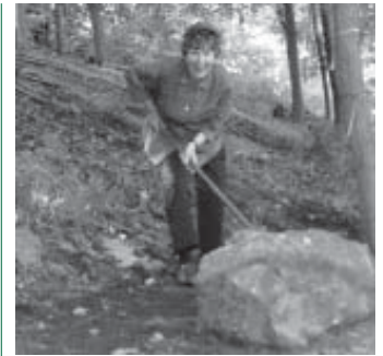
PIPC Executive Director Carol Ash joined a TC crew at work on the Twin Forts Trail.
