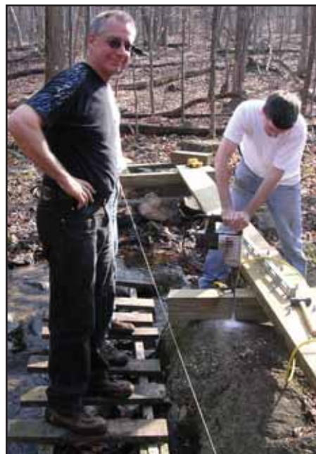
Scout Daniel Loughrey uses a rock drill supervised by Scout leader Frank Stevens.
