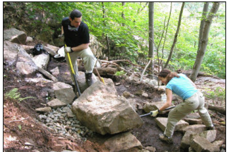
The AT restoration project at Bear Mountain, scene of the above rock moving activity, will include building an ADA-compliant path at the summit.
