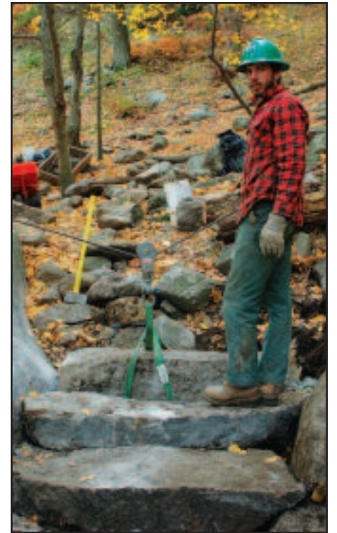
Crew leader Tom Kindling installing some of the first steps during year one.
