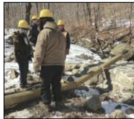
A bad pole broke before placement.
