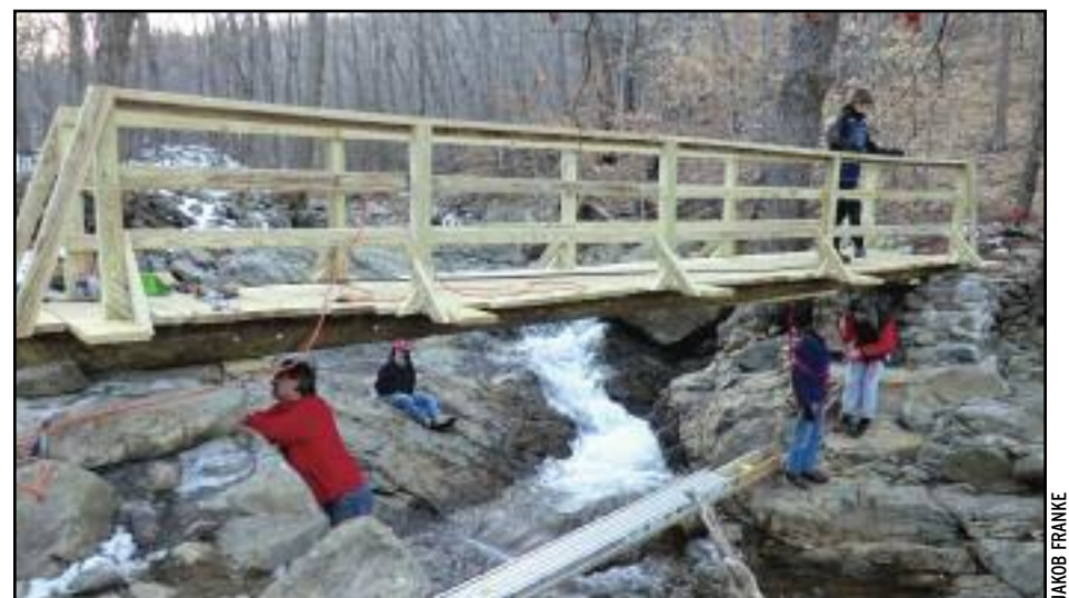
One new pole and two work trips later, the Scouts had successfully replaced the bridge. Thanks to all. Happy Hiking!
