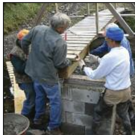
Long Path North Hiking Club bridge builders repair crossing at Tubbs Pond.
