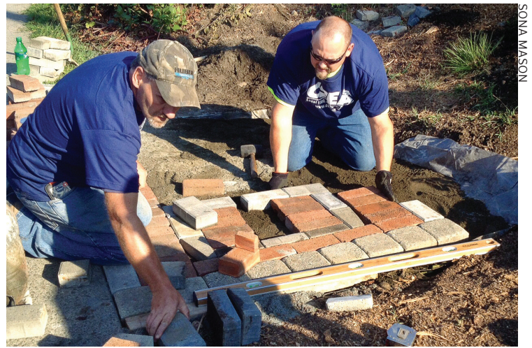
A crew from the Suffern Department of Public Works paved a welcoming entrance to the S-BM Trail in town.
