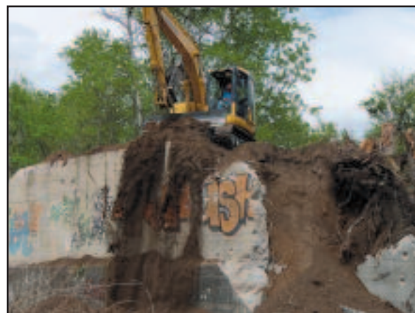
Andy Garrison is at the control of an excavator at the TC’s LaFarge site.
