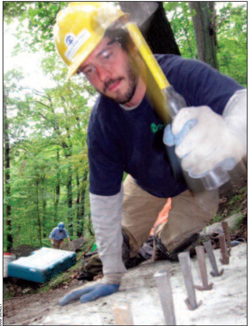
Appalachian Trail Conservancy Crew Leader Adam Daniel hammers wedges to split a rock at Bear Mountain.
