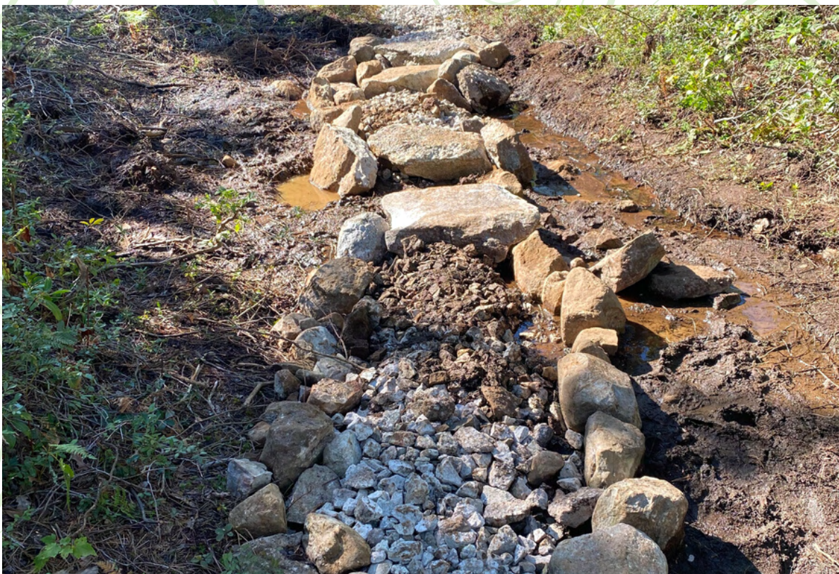
A section of the Mine Hole Trail where the stewards laid stepping stones in a wet section
